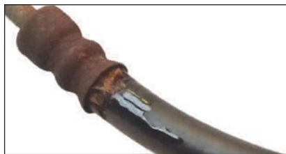
COMMON PROBLEM Leaking hose at collar
